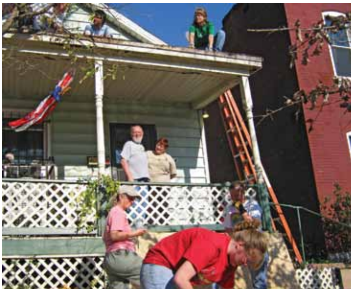
Jim and Diane Schmidt watch from their porch as volunteers repair the couple's roof as part of a neighborhood work day organized by Lutheran Housing Support in north St. Louis, Mo.
